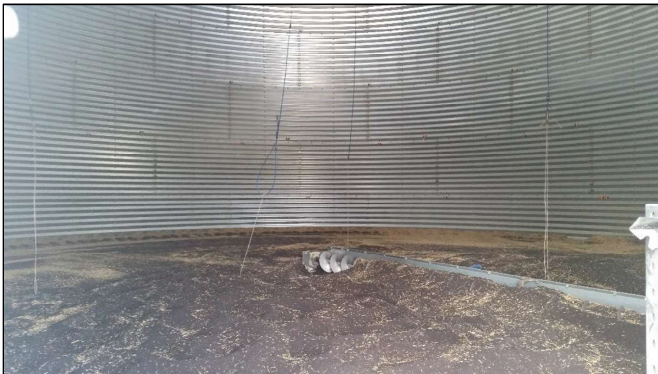
Figure 6. OPI temperature and humidity sensor cables.
