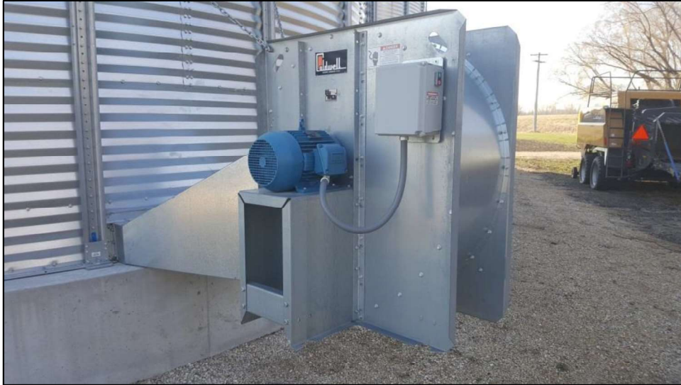
Figure 5. 10 hp Centrifugal fans.
